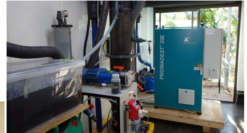
Nitrification reactor: Newlands Mashu, South Africa
